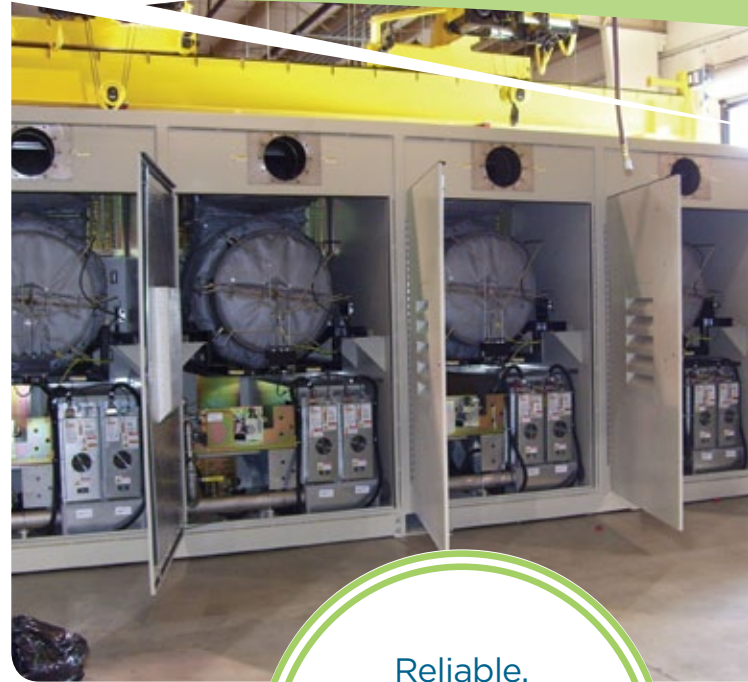
Capstone Micro-Turbine Generators
