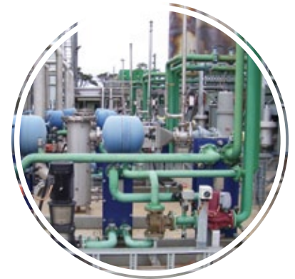
Methane-rich Biogas Treatment
